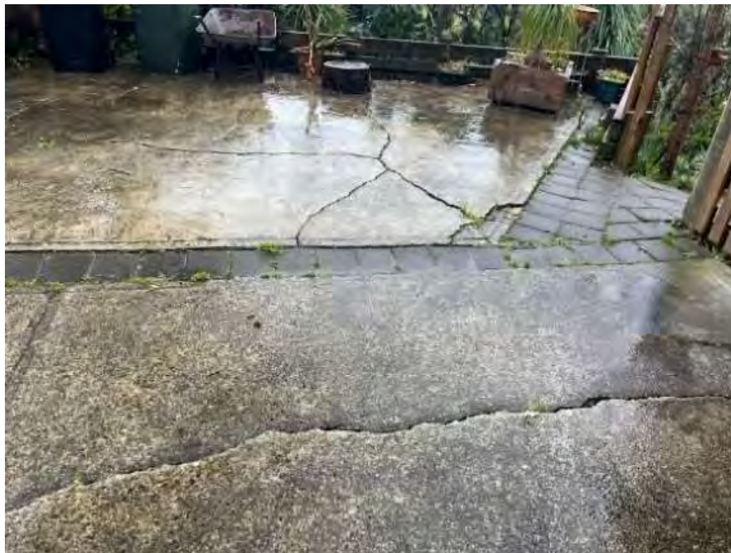
Figure 3: Cracks in pathing at my neighbours Tamaki Street property
