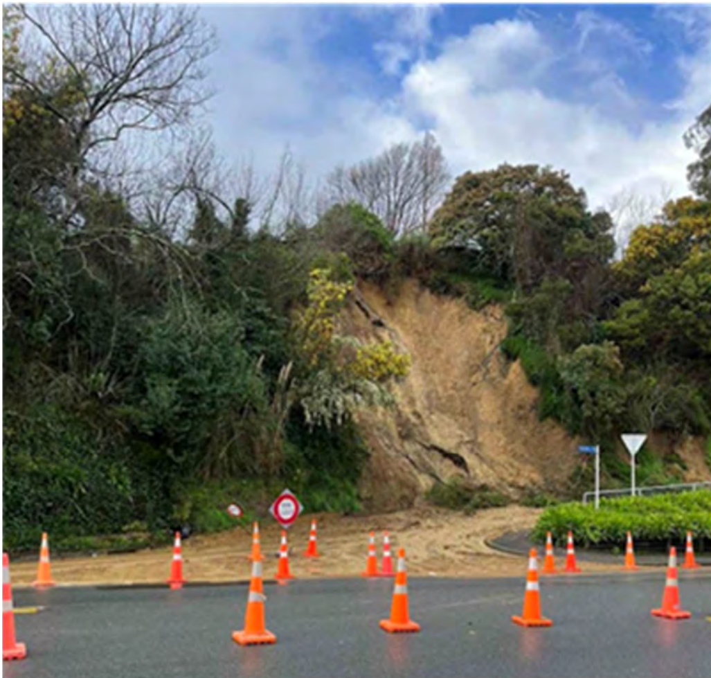
Figure 1: This property in Tosswill Road will be zoned high density suitable for 6 story apartments. The property has regular slips and has 2 hazard slip overlays.
