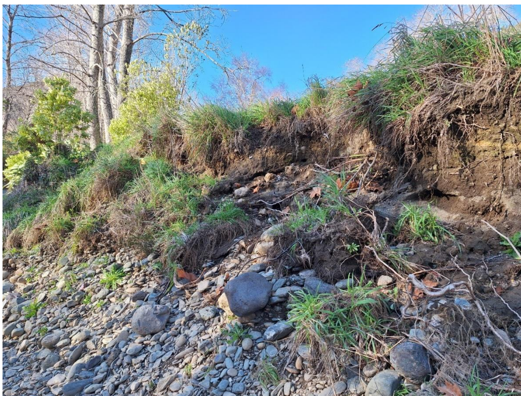
Photograph B.12: Area of visible scour on the true left side of the riverbank.
