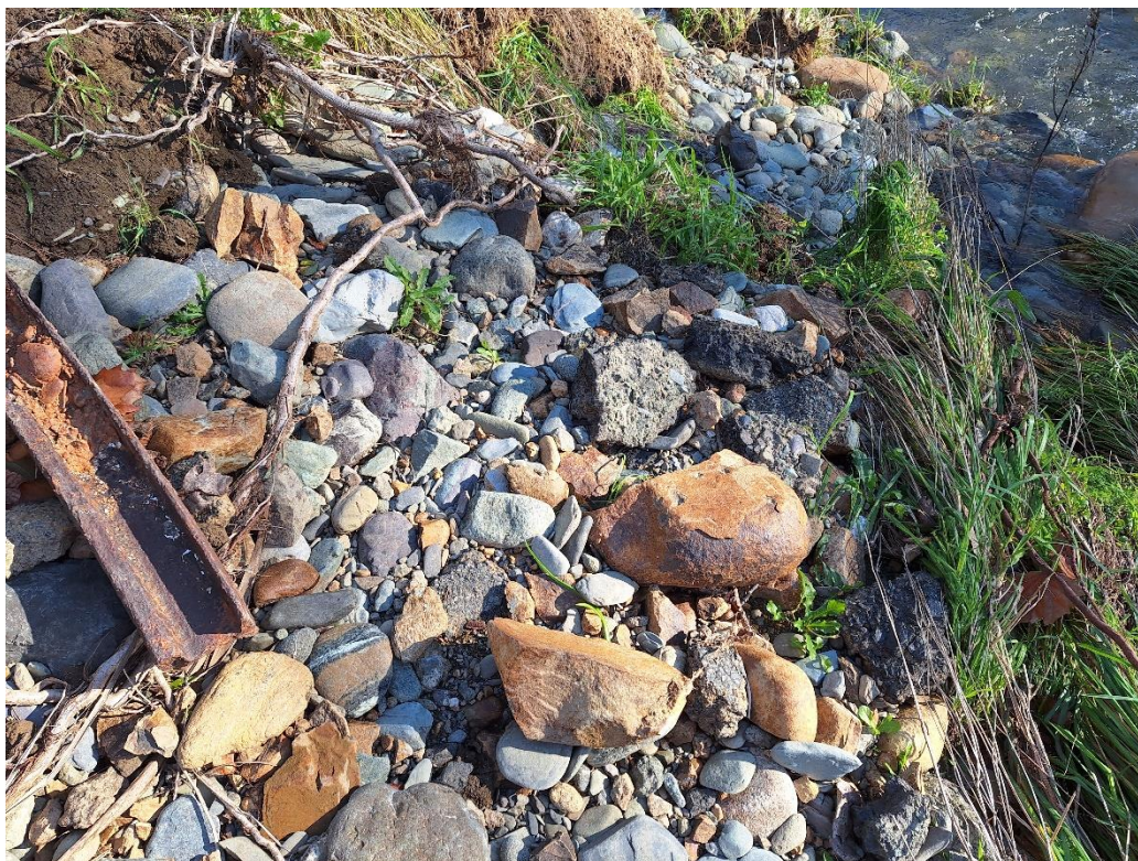
Photograph B.15: Rail material scattered on the surface of the scoured-out area.
