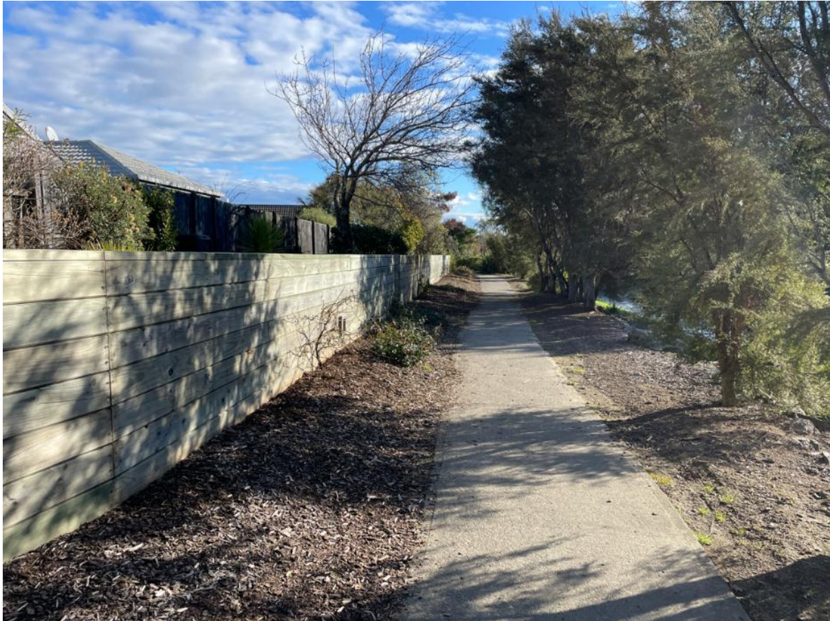
Figure 5.5: Example of pole wall floodwall along waterway in the Nelson region.
