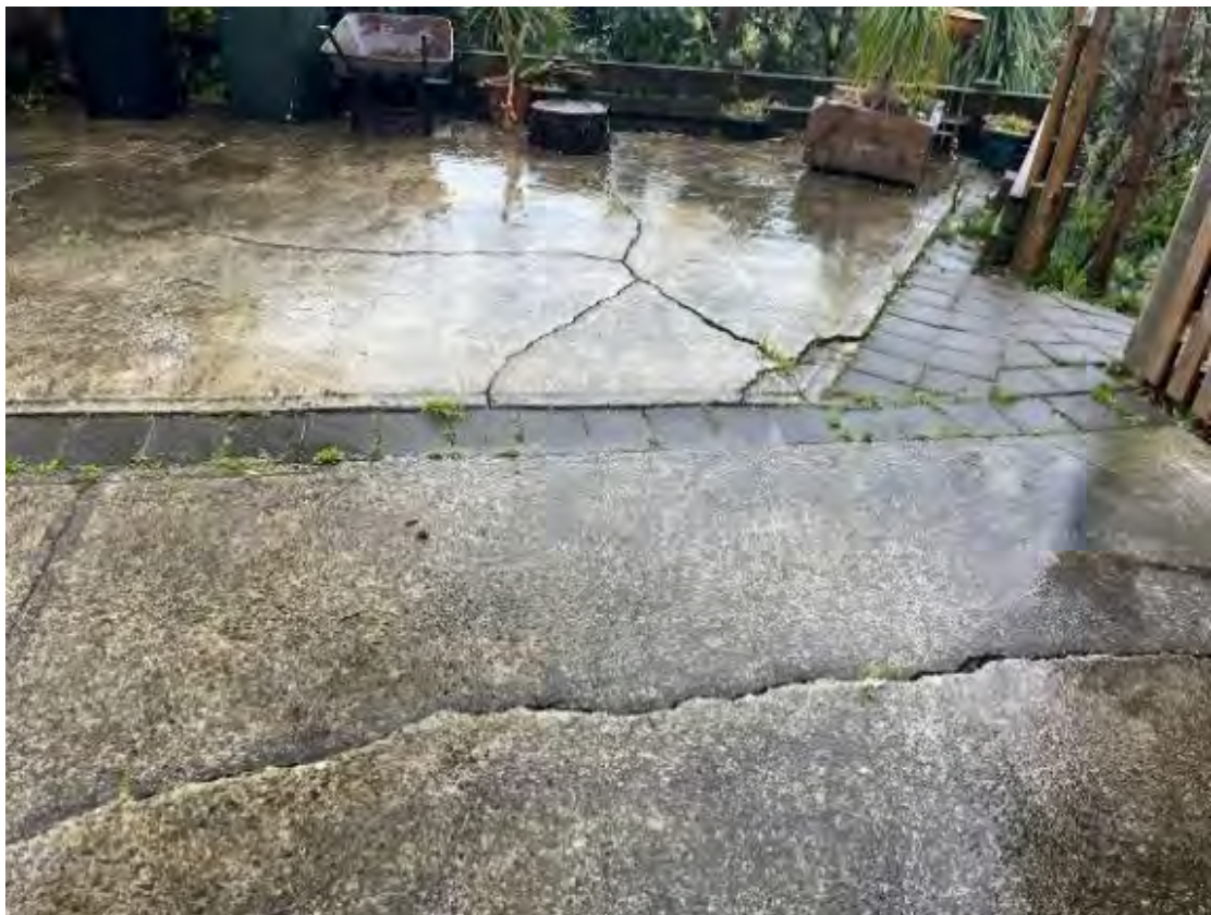
Figure 3: Cracks in pathing at our next door Tamaki Street property
